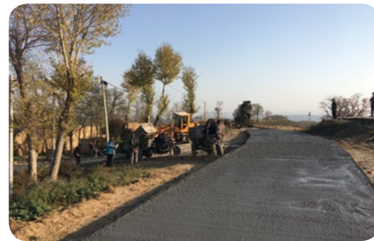
捐资修建古槐村通村路及巷道建设施工 Guzi Village is under construction via roads and roadways
