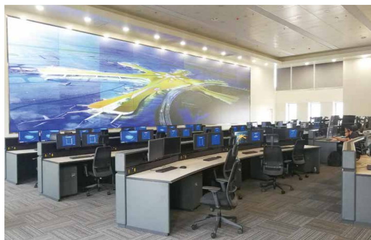
助航灯光和助航灯光单灯监控系统 Navigation lighting and the navigation lighting single-light monitoring system
